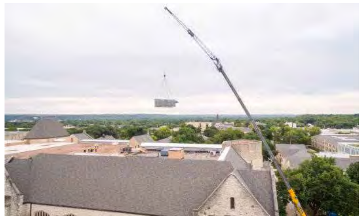
Three massive heating, ventilation and air conditioning (HVAC) units on the roof that were close to the source of the fire were deemed not salvageable, so they had to be removed.
