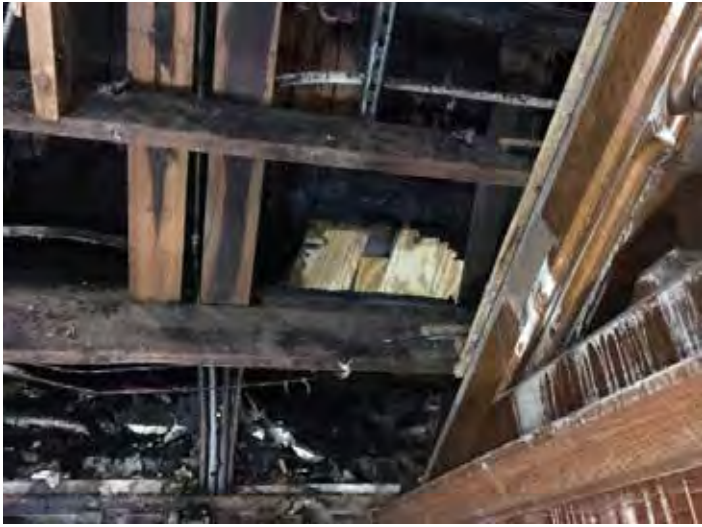
Charred, scary holes up close and personal in the ceiling that have been covered by a temporary roof.
