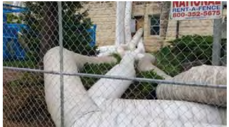
Dehumidification - Stabilizing Conditions Inside The Library
