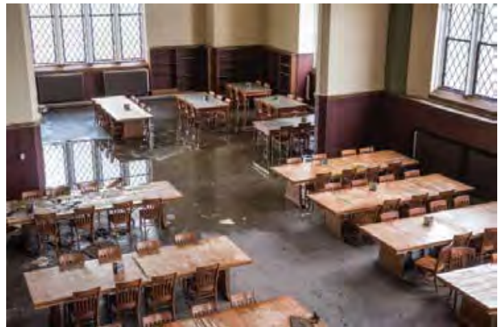
Water pooling across the floor and warped tables.
