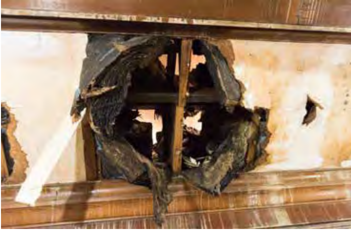
A hole in the Great Room ceiling.
